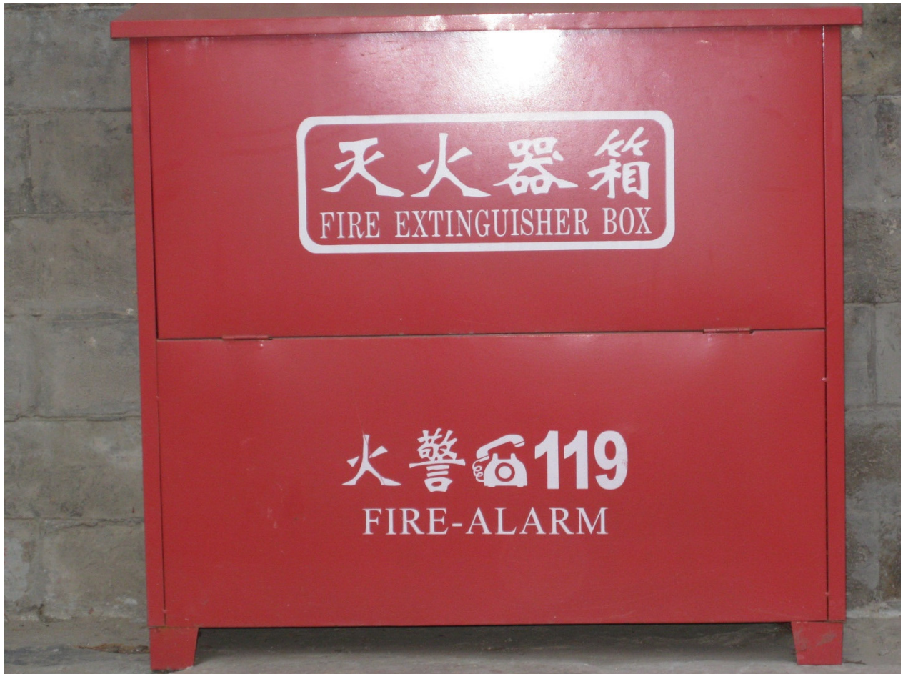
FIGURE 2 HERE. Caption: 'Fire extinguisher Box'
